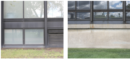
The articulation to the ground of both buildings differs and is a big part in their perceived lightness.
