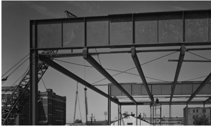
Construction of Crown Hall; the supporting girder forming the frame are clearly visible, as well as the roof purlins suspended to them.
